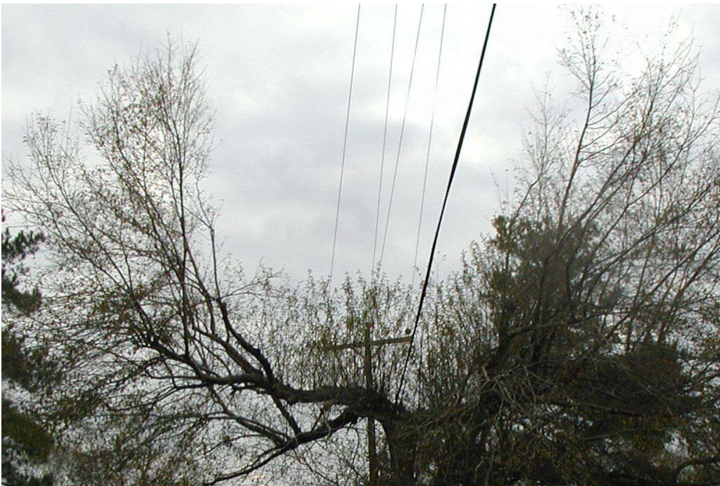
Photo 7. One-Year Re-Growth Due to Re-Trimming Under a Three-Phase Line
